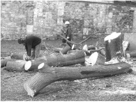
Removal of mulberry tree whose weight and roots threatened integrity of vault roofs.
