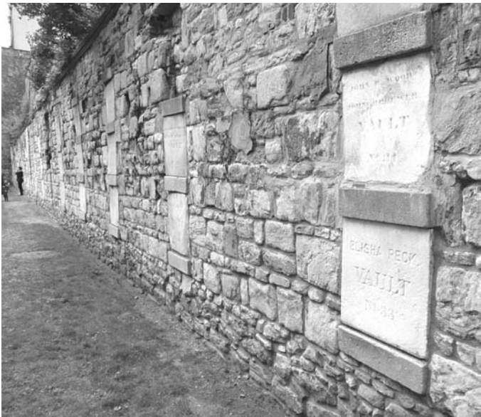
The South Wall of the Cemetery has been completely repointed this year from below ground level to about four feet above ground.
