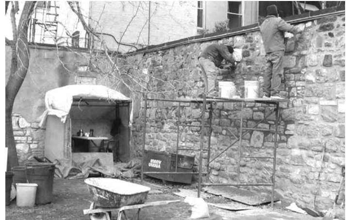
Masons repointing the East Wall and repairing problem spots, with their shelter from sun and weather at the left.
