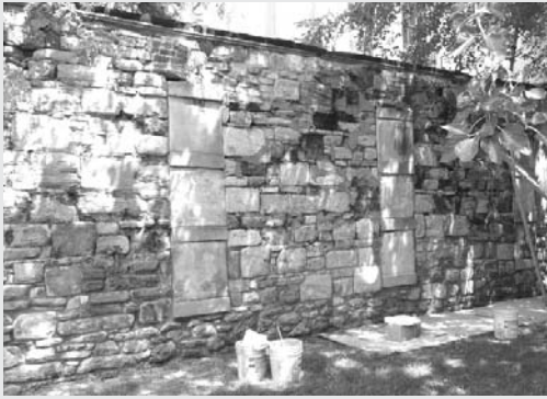
The existing eastern portion of the North Wall of the Cemetery with repointing work in progress.
